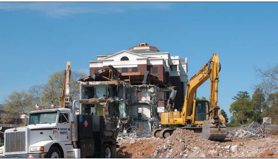
Last vestiges Demolition crews last week finished leveling Noble Hall, the final residence hall on the north end of campus. A transportation technology center for the College of Engineering will eventually occupy the site. Behind the last vestiges of Noble Hall is the College of Business.
