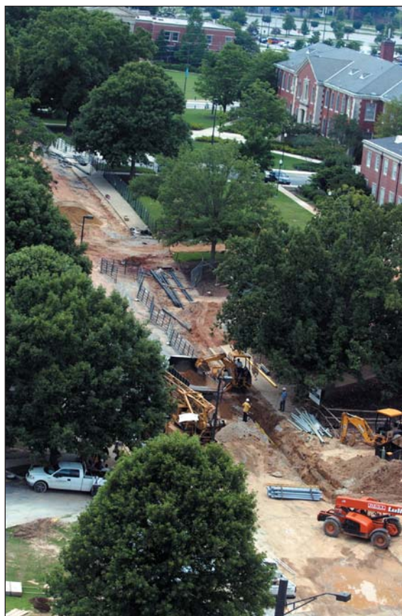
Infrastructure Workers install lines under Thach Avenue for AU's central heating and cooling system. This section will carry traffic again when the work is completed, but a section of Thach beyond the bottom of this photo will be converted into a pedestrianway.
