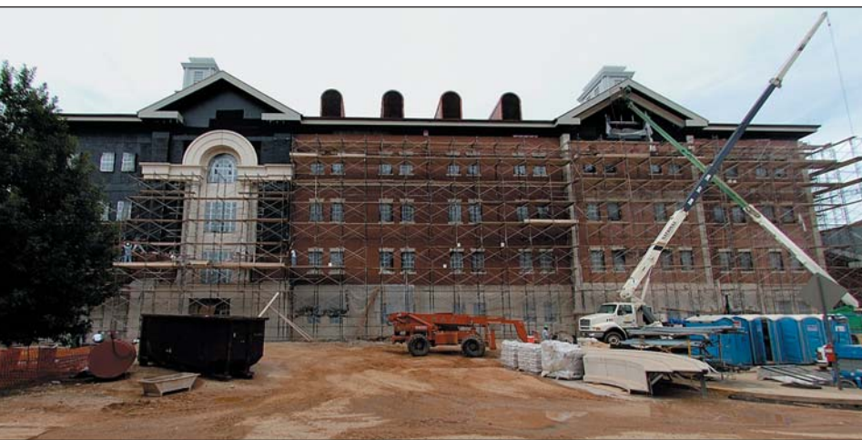
Brick by brick Construction workers are applying a brick exterior to the largest of three buildings in AU's new Sciences Center. Many core curriculum subjects will be taught in the complex, which will house laboratories, classes and offices for the College of Sciences and Mathematics and science-related disciplines in other colleges and schools.
